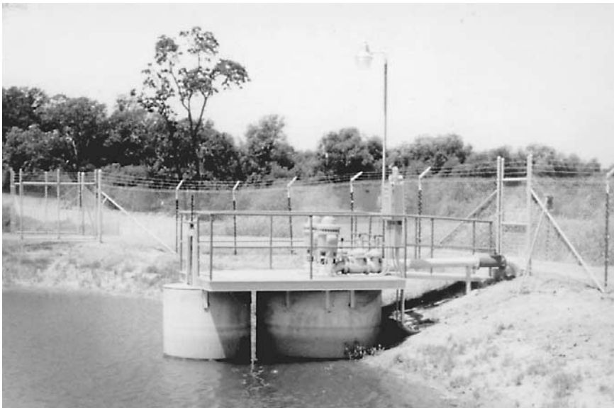
Figure 9.2 Distribution pumps in the side of a storage pond dike.
