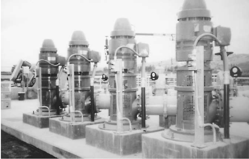
Figure 9.1 Typical outdoor wastewater pumping station.
