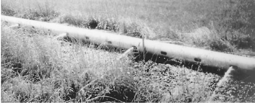
Figure 9.5 Typical gated pipe distribution unit.
